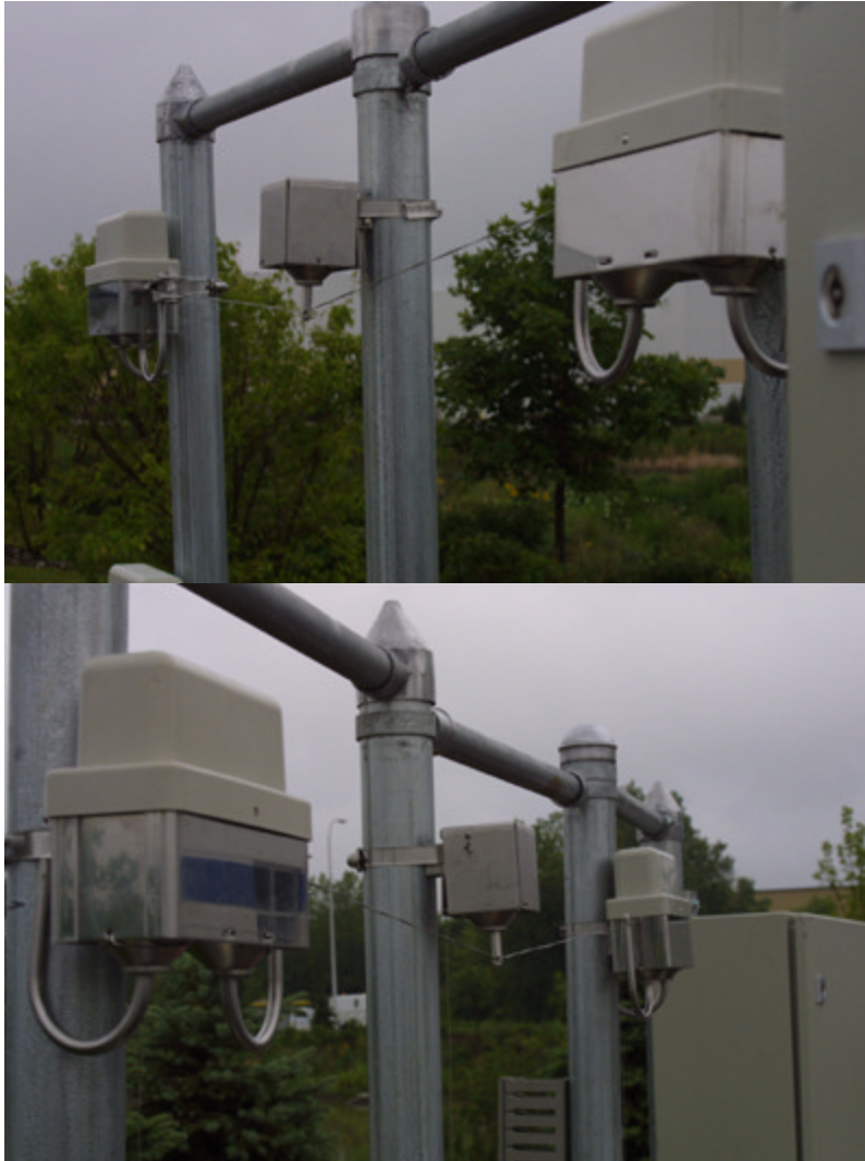
Figure LSS+4048 An E field system by Siemens creates an electronic barrier through a series of parallel wires across the fence line.
