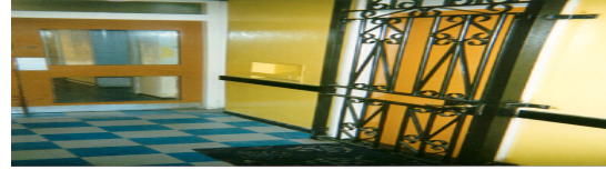
Figure LSS+3222 External - Heavy duty right hand outward opening steel gate proud of building line with single lock and no cover plate; Internal - Right hand inward opening timber door, locks unseen.
