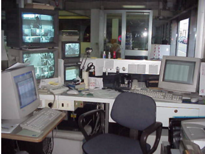
Control room of Diamond Center.
