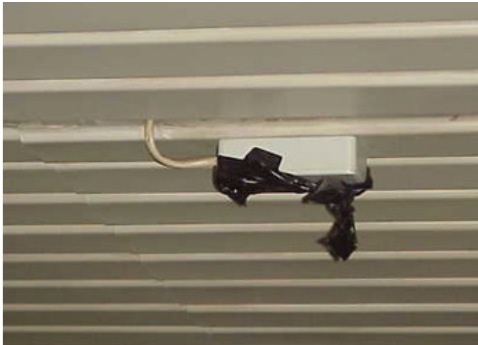
Light sensor, mounted in strong room.
