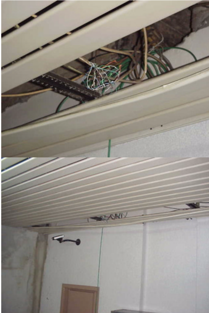
Cabling in an adjoining room were spliced into.
