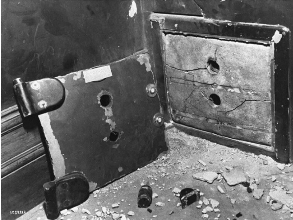
Figure LSS+3535 Shown (right) is a burglary where it is suspected that a drill rig caused the fracture of the outer skin of the door. In the photograph (right) a core drill was utilized.
