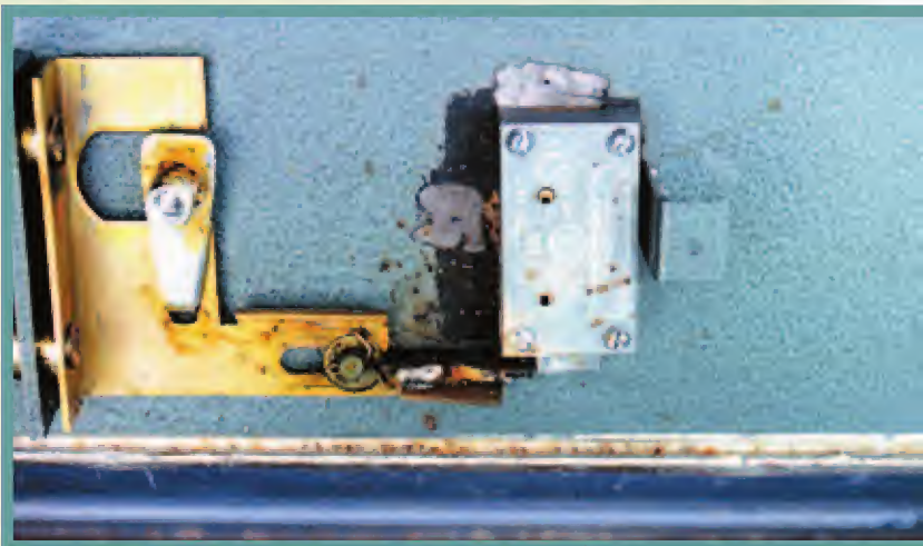
2. Inside view of previously repaired door. Note weld marks on bolt bar.
