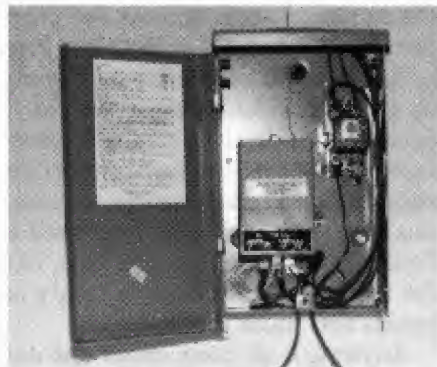
9. The alarm's control box.
