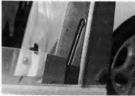
3. Bolt is placed on the glass to keep window following this track, preventing easy tool insertion.
