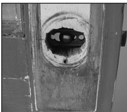
1. The hole in the door is cut wrong.
