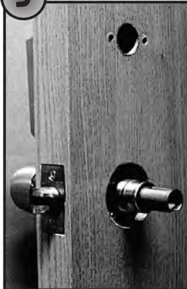
The latch has been installed and the front lock unit with chassis is in place.
