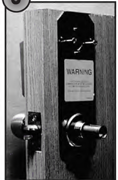
The reinforcing plate is positioned and the mounting screws have been partly tightened.
