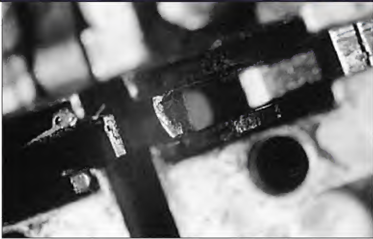
12. See the damage caused to the lock body that absorbed the pressure from the bolt actuator.
