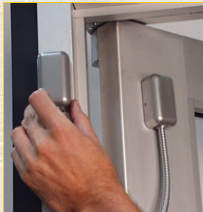
16. Wiring was run through a wire transfer cable attached to the door.
