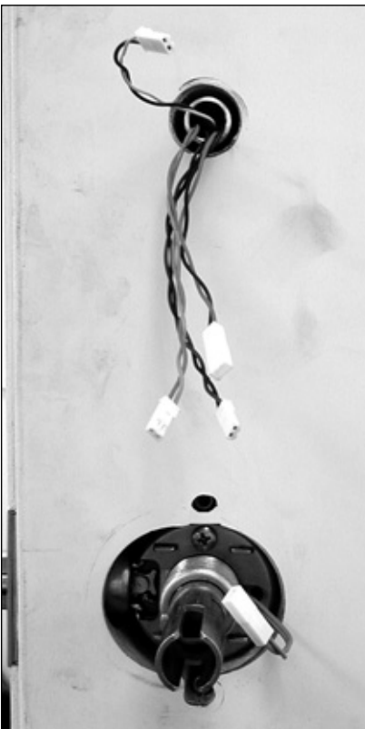
5. With all of the holes drilled, the outside housing and lock assembly can be slid into place.
