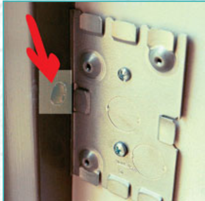
5. The arrow points to the entry hole in the highlighted area of the frame. This hole is for the cable of the DK-26 Touch Pad to enter the building. Note the mounting plate for the Wire Mold junction box.
