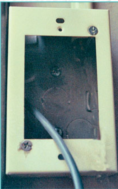
7. The cable enters through the frame and into a Wire Mold junction box that has been secured to the mounting plate.
