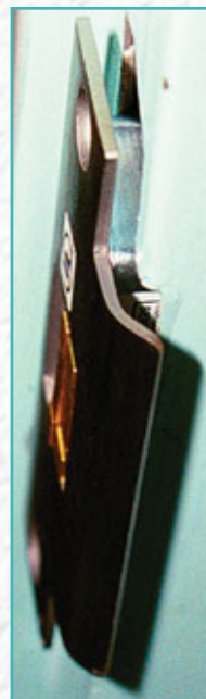
32. Securitron's UNLATCH being placed in the expanded strike opening. The wires, of course, have already been run up the frame and into the Panduit Junction Box.
