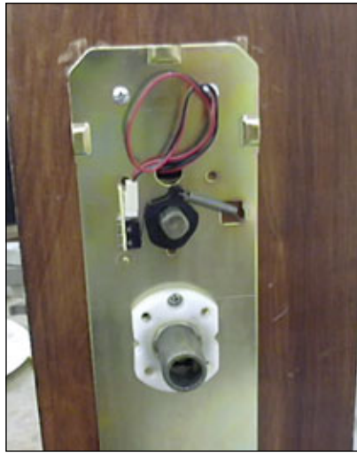
30. Tesa remounted to door. Two top screws and two screws through the plastic at the spindle. Extra wire is coiled up to stay out of the way. Take special note of the deadbolt switch. If installed wrong, the card will not operate the lock. Try the lock with the door open the first couple of times. The switch tells the lock that someone is in the room and not to allow entry by the maids or other normal cards. The manager override card or the hand held module could still open the door.
