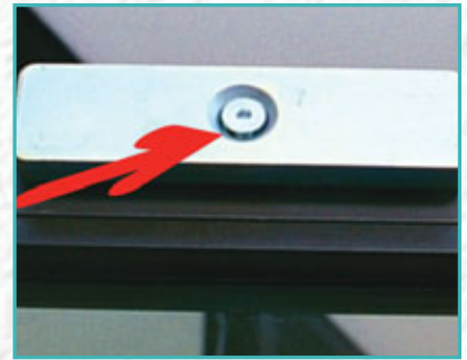
19. This is a Model 32 strike plate on a narrow-stile, store front door. The red arrow points to an obvious gap between the through bolt and the strike plate. The strike plate needs to flex so that when the door closes, the strike plate automatically aligns with the magnet to provide the maximum amount of security to the door. NOTE: The Model 32 is used as a traffic control lock and not a security lock. If the possibility of aggressive attack exists, then the lock used should be either Model 82 (1800 pounds of force) or a Model 62 (1200 pounds of force). Of course, on a glass storefront door, there would be little reason to have anything more secure than a Model 32 (600 pounds of force) since the glass could be broken easier than the lock could be forced open.
