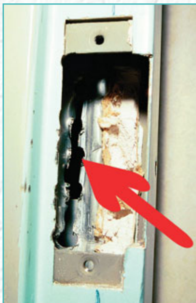
31. Note that the wall construction is metal studs with wallboard over them. The arrow points to the holes that I drilled to remove much of the stud material and then, I simply used a rotary cutter to finish the cutout and remove the wallboard.
