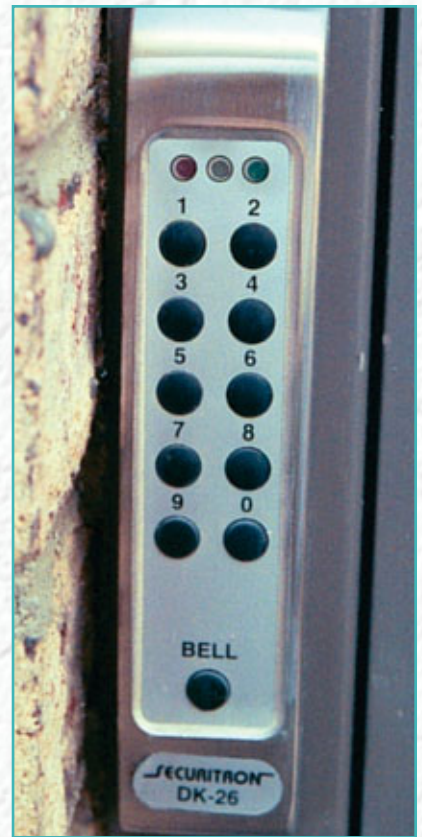
6. Here the DK-26 is mounted to the outside of the frame with the wires going through the frame to the inside of the building.
