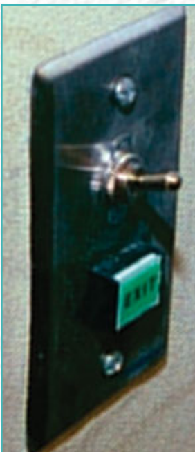
21. The switch shown here is Securitron's SEPB3. This switch is mounted behind the counter of the customer entrance area of a pizza delivery store. The switch is used to "buzz" folks into the store after dark. The toggle switch that you see over the pushbutton on the SEPB3 is the on/off switch for the Maglock. When the toggle is in the off position, simply pulling on the outside handle will open the door. Once the switch is in the on position, the Maglock activates and customers have to be "buzzed" in.
