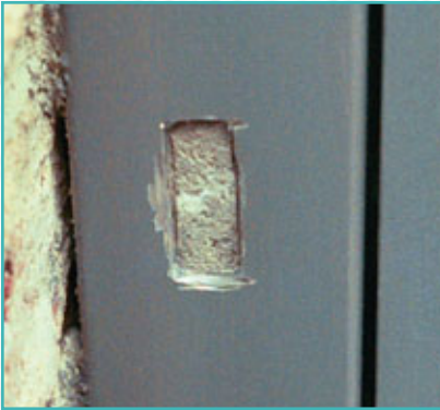
4. This door is the employee entrance to a church. The hole you see in the frame has been cut with a Dremel tool to make it easier to drill through the concrete and penetrate the interior of the frame prior to mounting a Securitron DK-26.
