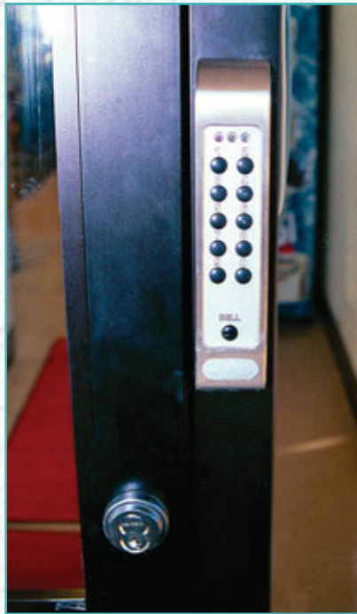
25. This is the finished installation on the driver's door. The DK-26 touch pad is installed. Behind the touch pad is the internal exit switch. Note the KEYMARK Mortise cylinder for securing the door after closing. The customer pickup area is to the left of this door. The AR lock has a dummy cylinder on the outside and a thumb-turn on the inside for after-hours security.
