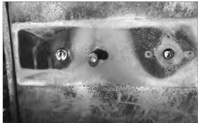
2. The melted dial and handle were removed, notice that the key lock has also melted.
