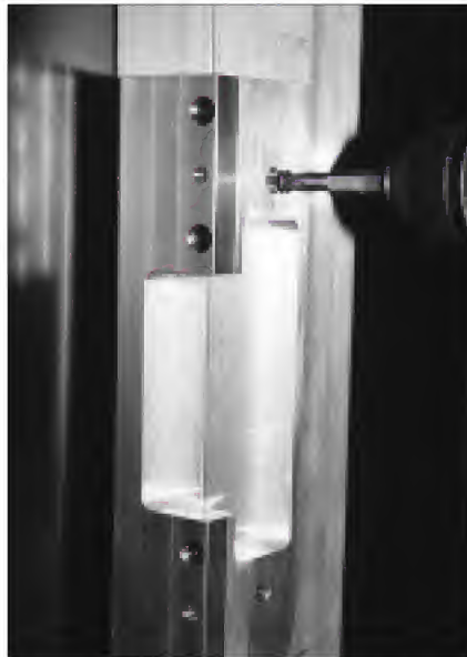
10. Use the self drilling drywall screws to attach the template to the frame.
