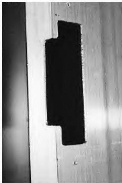
11. The finished cut includes holes for attaching the U-Tabs needed for mounting the electric strike.
