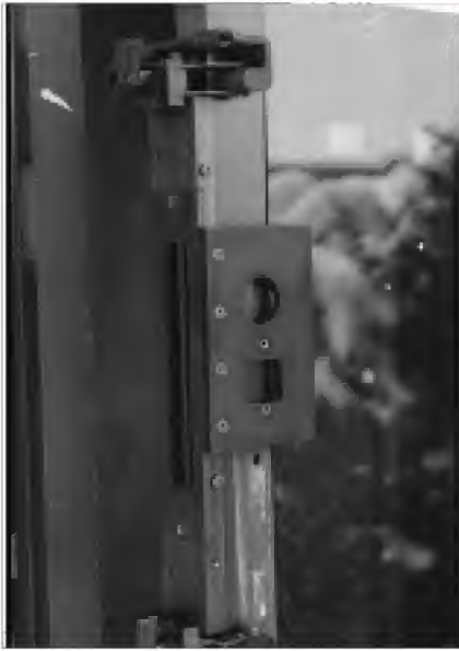
5. After removing the existing push bar and pull handle, the HIT-45 is clamped to the door and ready for cutting.
