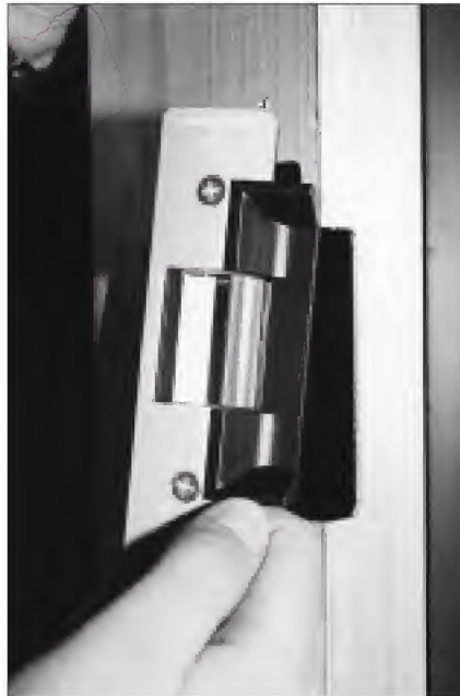
12. After checking for the initial fit, the U-Tabs were installed and the strike mounted to the frame.
