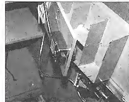
13. Mounted locks showing cables.
