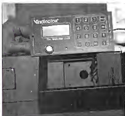
8. Vindicator panel and back up 6 volt battery ready to be installed
