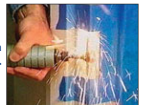
9. An ANSI dust box portion will need to be removed.
