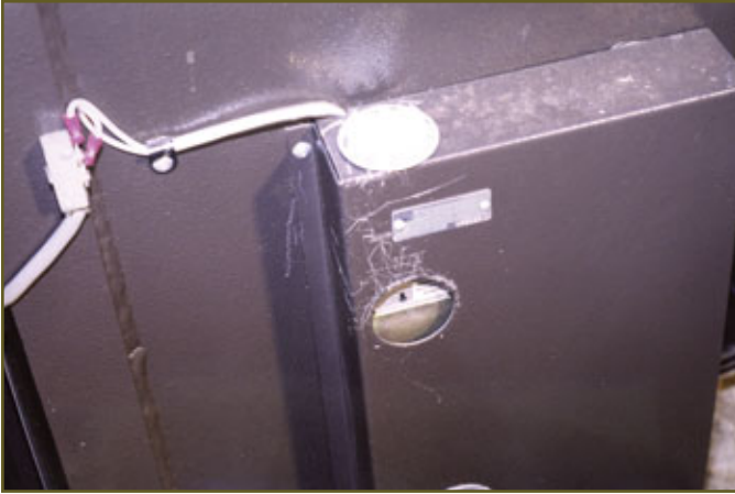
3. Key cover button removed. Scratch marks above hole.
